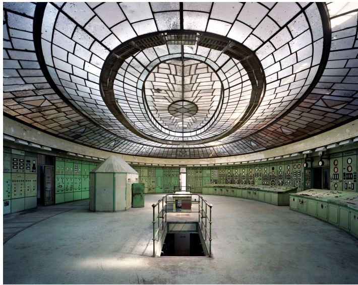
Control Room, Kelenfold Power Station, Budapest (2012)
